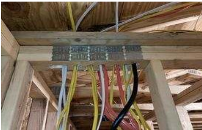
Wiring in the Abbey
